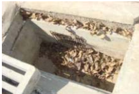
Figure 3: Drainage inlet at the Presidente Carlos Luz Av: deposits of sediments and other debris
